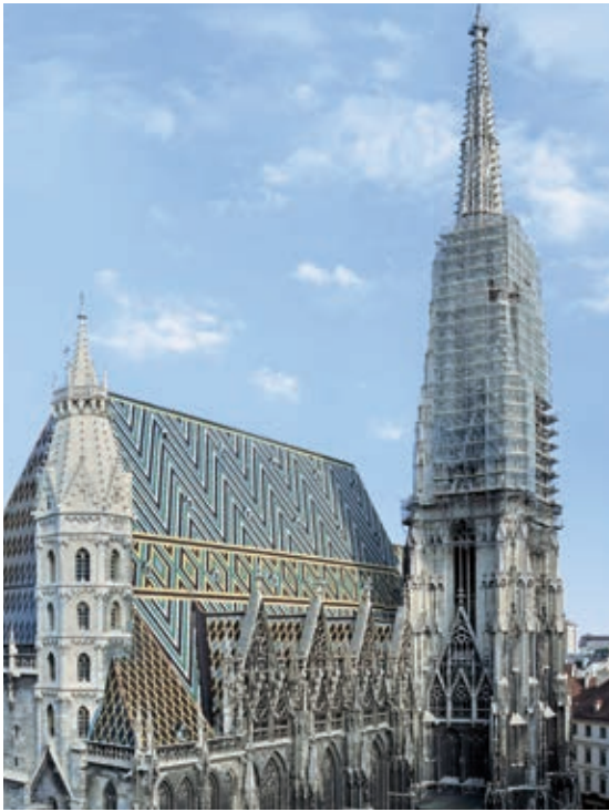
We used a bespoke modular scaffolding system for St. Stephen's Cathedral in Vienna which was erected around the building without the use of anchors
