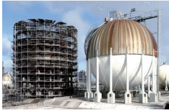
XERVON also provides top quality logistical services when spherical tanks need to be serviced – supplying the enormous volumes of material needed to erect work platforms and protective scaffolding around the huge surfaces
