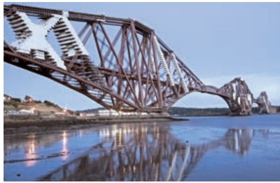
Erecting enclosed scaffolding around bridges whilst traffic continues to flow without interruption – such as during the Forth Rail Bridge project in Scotland – is just one of the many international tasks we are able to master
